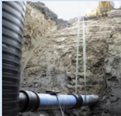
The connection to one of the many chambers on the pipe. The components are being joined by electrofusion.
