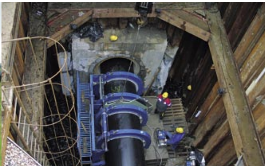
Installation of dia. 1,400 mm PE pipes in the pit under Czerniakowska St.
